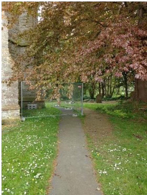
The footpath around the Church Tower Fenced off due to falling masonry.
